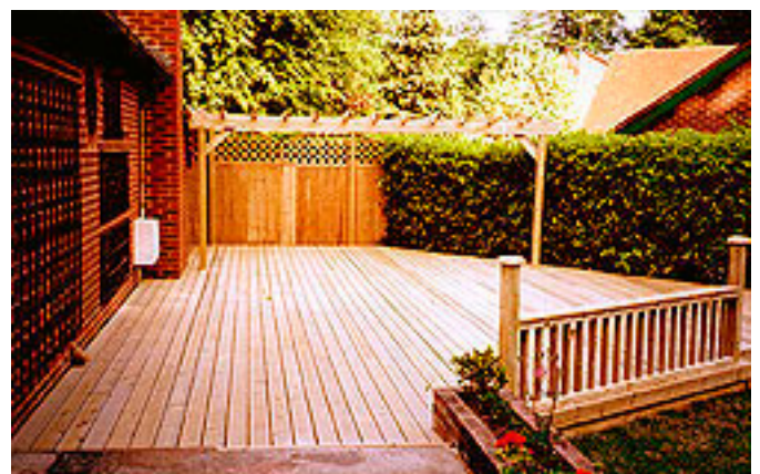
A treated-timber patio deck is an economical and practical way to gain extra living space while simultaneously enhancing the home landscape.
