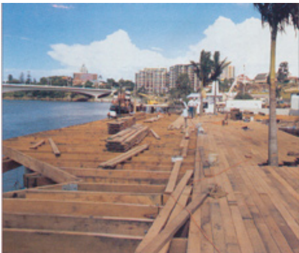
Expo 88 boardwalk under construction using hardwood substructure and 45 mm thick hardwood decking.
